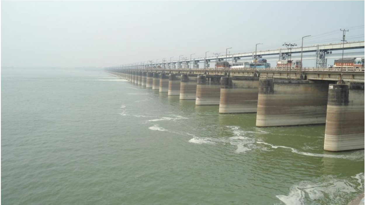
Image No 20 : The Farakka Barrage, Farakka. The Farakka barrage has been blamed for worsening land erosion by the Ganga. Source – India Climate Dialogue
